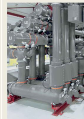
TC PSEM installation externe
